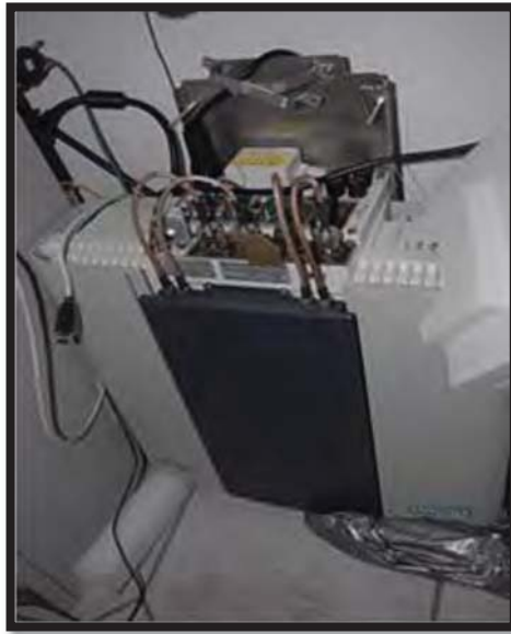
Figure 2.1: Base Transceiver Station
