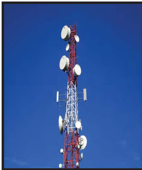
Figure 2.2: Base Transceiver Station Tower
