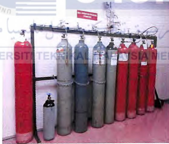
Figure 3.3: Hydrogen tank system
