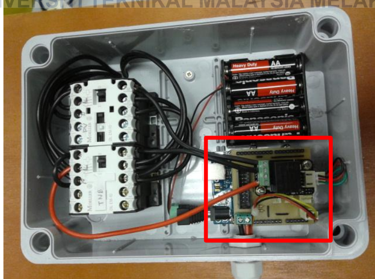
Figure 4.8: The PCB board with the arduino inside the box.
