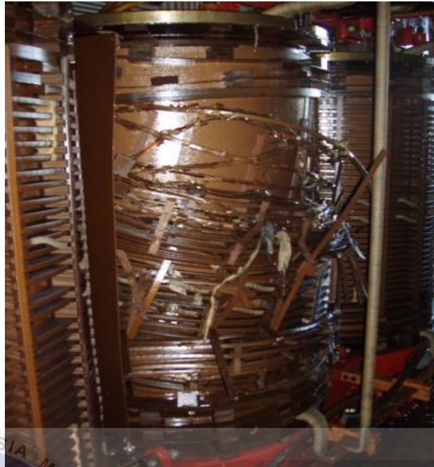
Figure 1.0: The transformer experienced mechanical faults [2]
