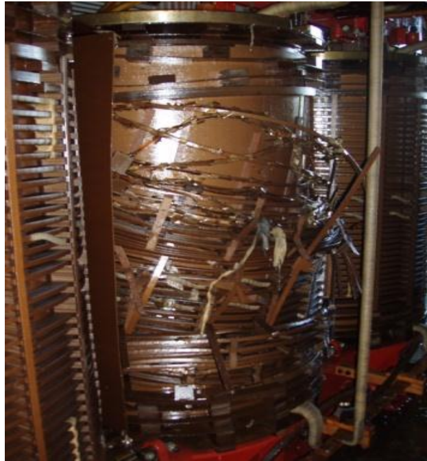
Figure 1.0: The transformer experienced mechanical faults [2]
