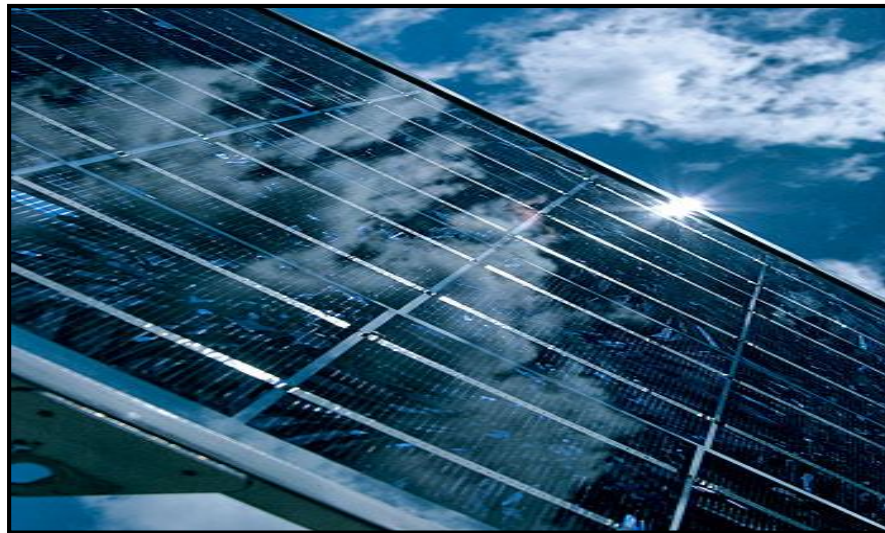
Figure 2.5: Clean solar panel.
