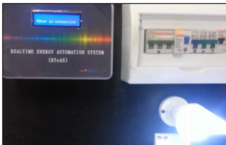
Figure 4.14: System reconnected the supply to consumer.
