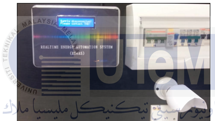
Figure 4.10: Smart Meter System disconnected the supply to consumer
