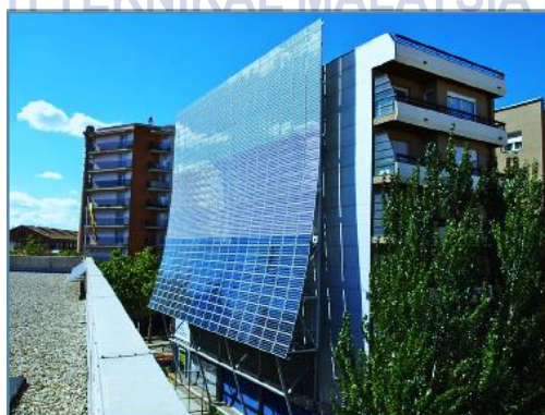
Figure 2.1: Photovoltaic solar panels [5]
