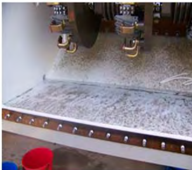
Figure 2.13: Free water found inside the new on-load tap changer [7]
