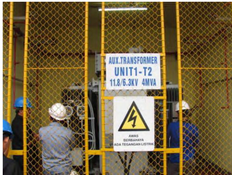
Figure 2.2: Auxiliary Transformer under Test [8]
