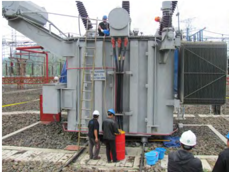
Figure 2.1: Main Transformer under Test [8]
