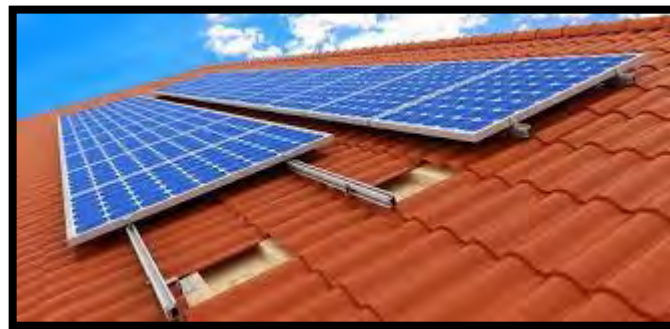
Figure 2.4: Roof Mounting System
