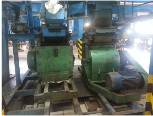
Figure 1.2 Ripple mill machine design in kernel recovery plant
