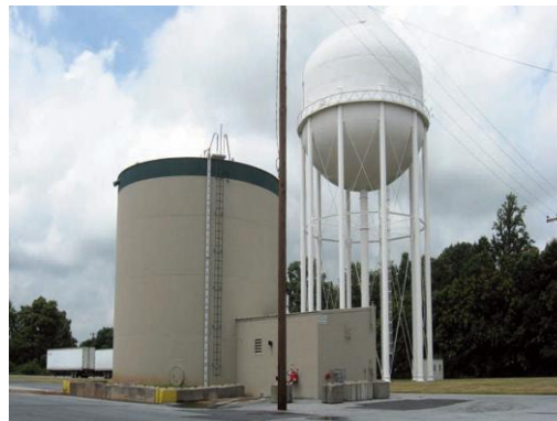
Figure 2.2: The fire water storage tank (Walter, 2012)
