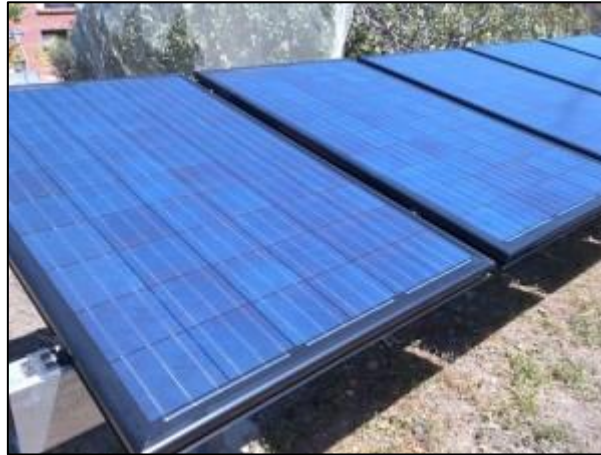
Figure 2.2 Poly-crystalline PV panel
